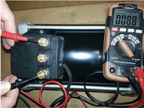
Figure 14 U and W terminal
