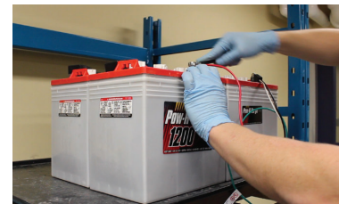
Figure 8: Reattach the positive lead to the positive terminal after disconnecting AC power.
